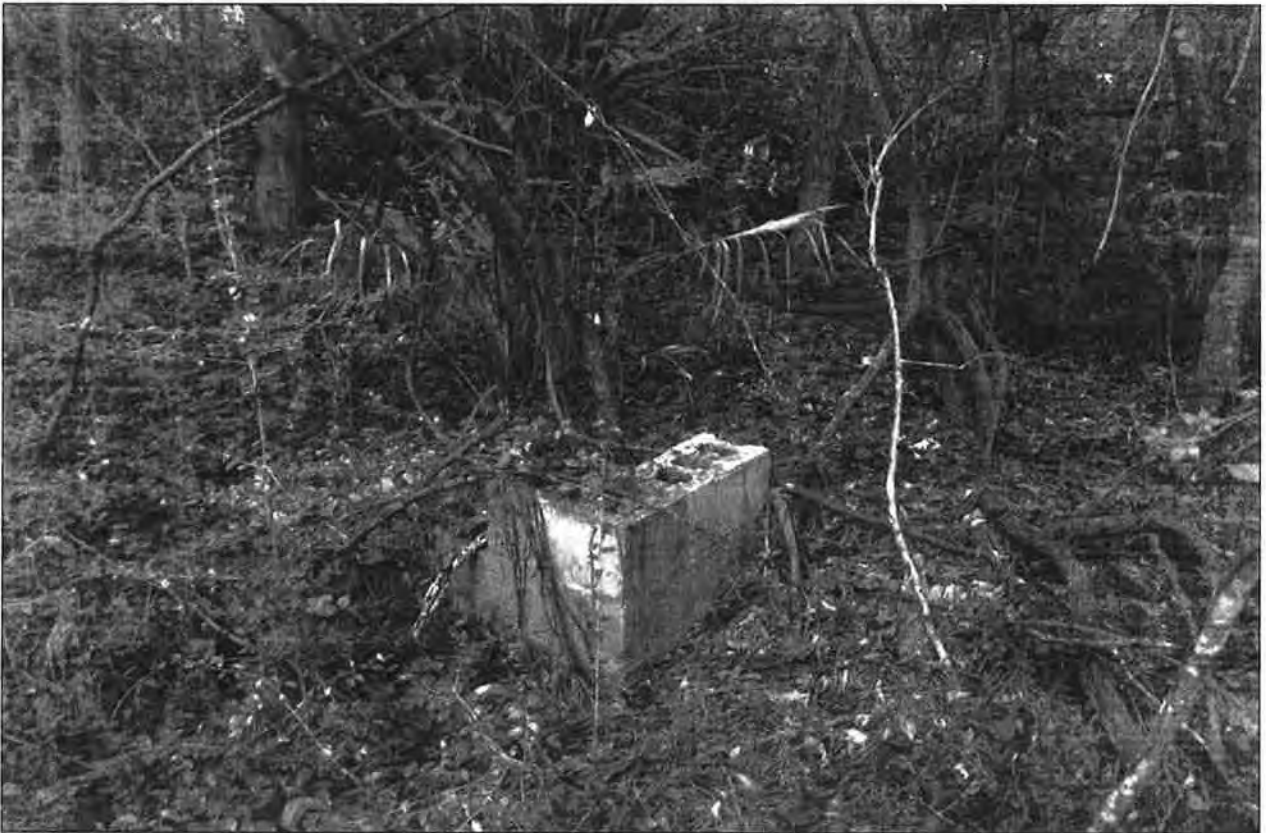
Figure 3.3 Views of the chimney (top) and foundation (bottom) surface features found at 38CH2645.
