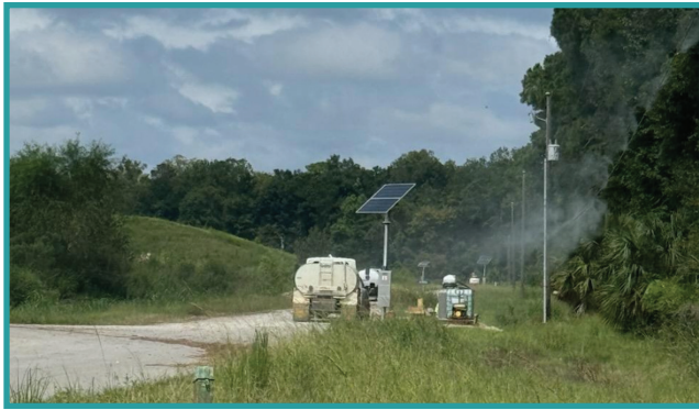
Perimeter odor misting system located at the Bees Ferry Landfill
