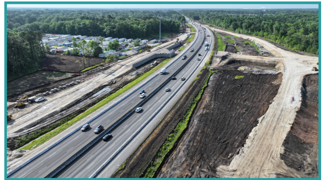
Substantial work has been completed at the Palmetto Commerce Interchange , another major TST funded project.
